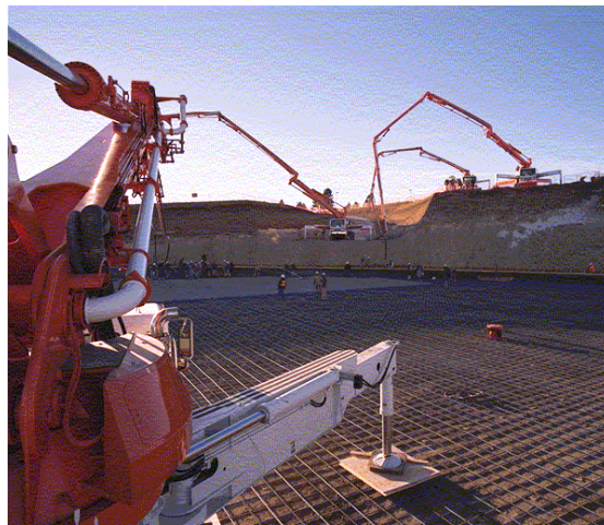
Foothills Water Treatment Plant 25 Million Gallon Storage Tank
